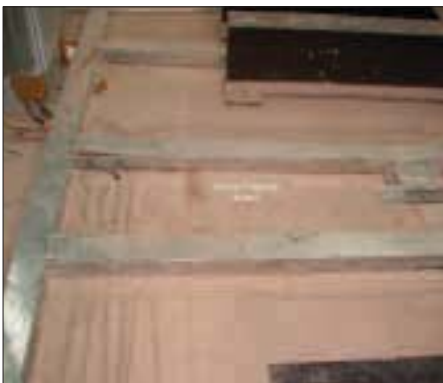
Machine-room trough – a serious tripping hazard
