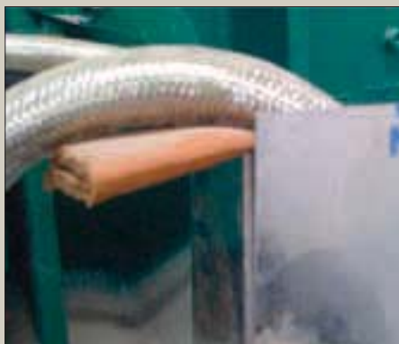
Wiring done imperfectly
